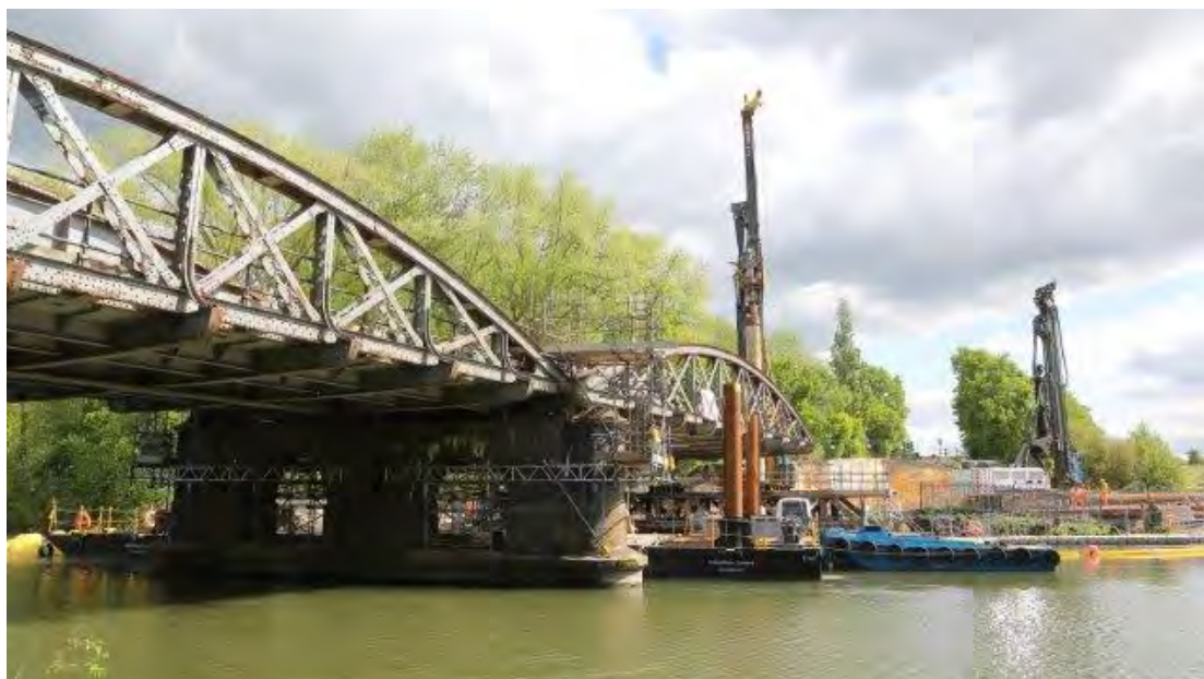
Work progressing well on 15th May as seen from the right bank towpath with piling in progress. Whilst the south span appears to be unsupported it is actually being held up by staging supported by the cylindrical piles.
