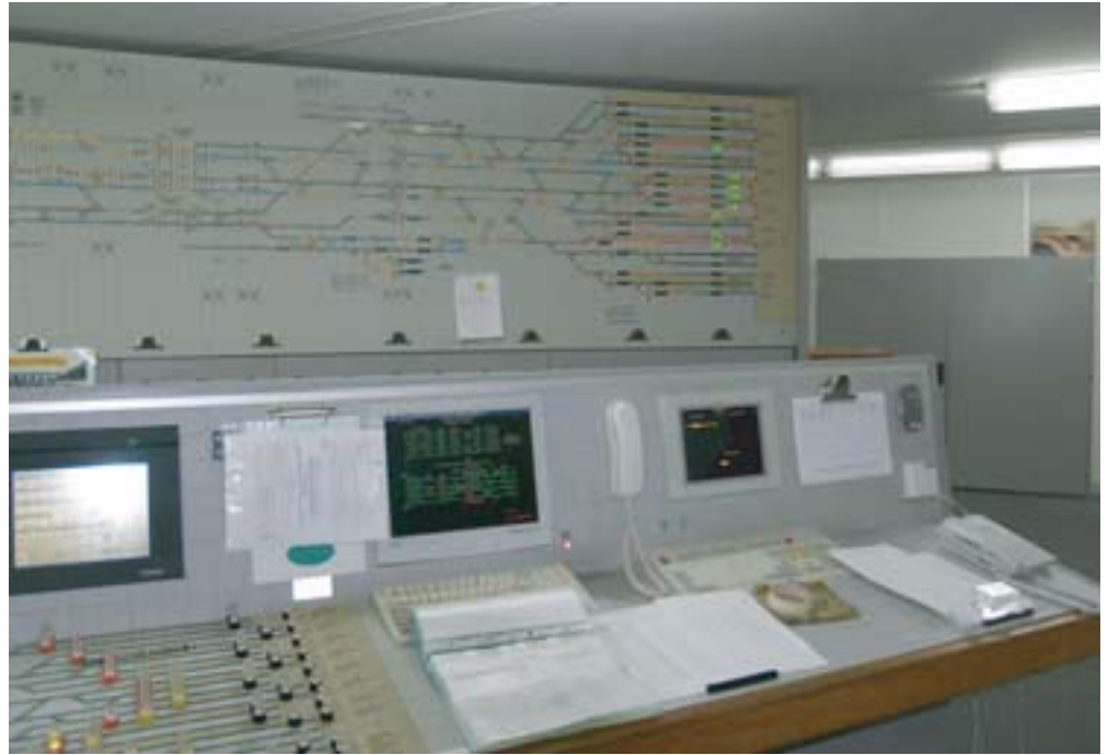
ABOVE: The Euston station end of the WM panel. The panel with the route setting button is at bottom-left. The monitor in the centre shows the line north of Hatch end to Watford Junction station (which has its own SCC) giving the signallers advanced warning of what is approaching.
