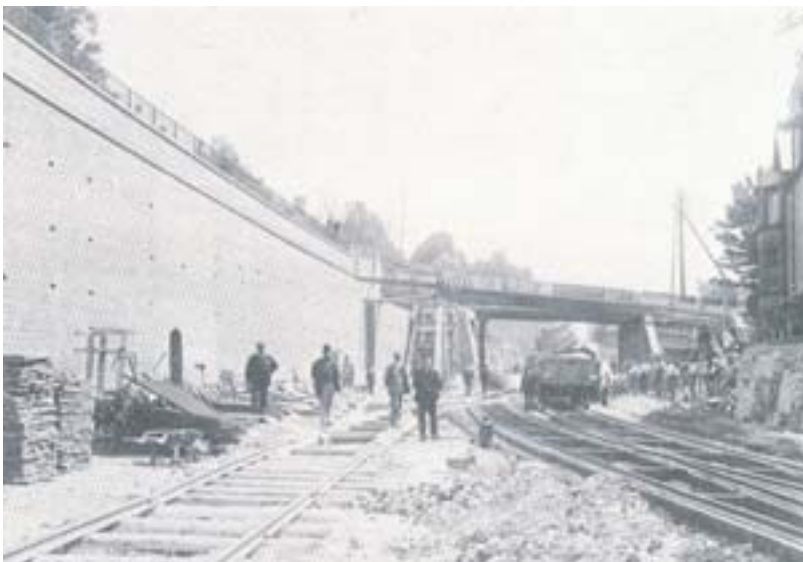
High Wycombe during 1904. The new retaining walls have been completed and demolition is about to begin of the second Wycombe Railway station, just visible through the Amersham Hill bridge, itself due to be replaced as part of the works.
