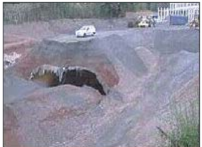
The tunnel immediately after the collapse. Note how the fill has been piled on top not equally at each side causing the arch to deform.
