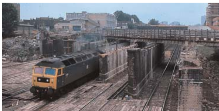
With work in progress to raise the bridge carrying the North London line clear of the impending overhead power lines, 47 502 approaches West Hampstead Midland, 18 August 1979.
